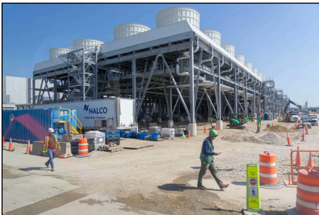
Heat-exchange fans help keep computer equipment cool at the Microsoft data centre in Mount Pleasant, Wisconsin, on September 18, 2025. Mike De Sisti/Milwaukee Journal Sentinel/USA Today Network/Imagn Images
